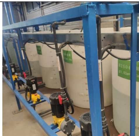
污水处理站加药区
